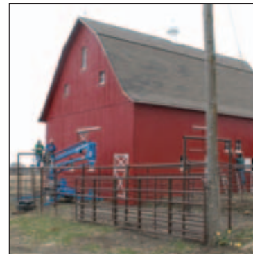
FINAL RESULT: Local FFA volunteers gave Gary Cotterill's 80- to 100-year-old barn a new coat of paint and installed new windows and doors.
