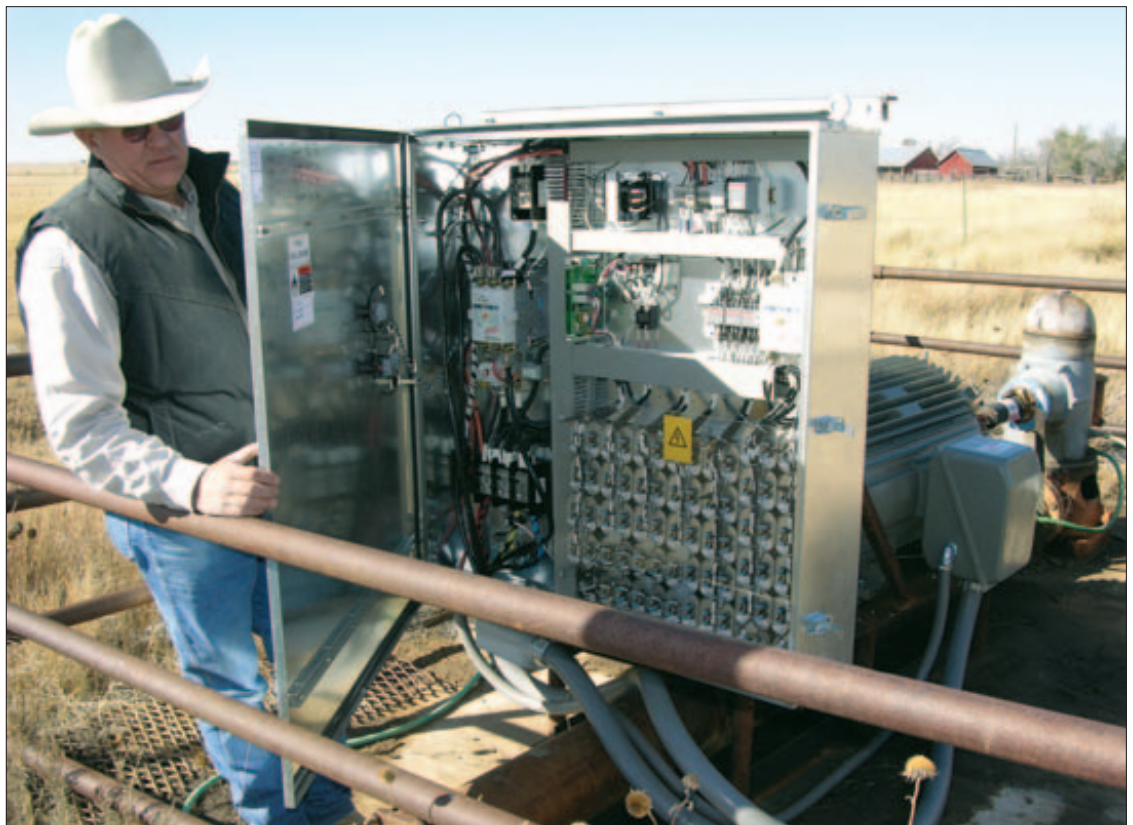
EFFICIENCY TECHNOLOGY: This bank of capacitors and the computer control module inside the box is part of the technology that helped Sowers use single-phase electricity to save over $11,000 in energy costs on this well last summer.
