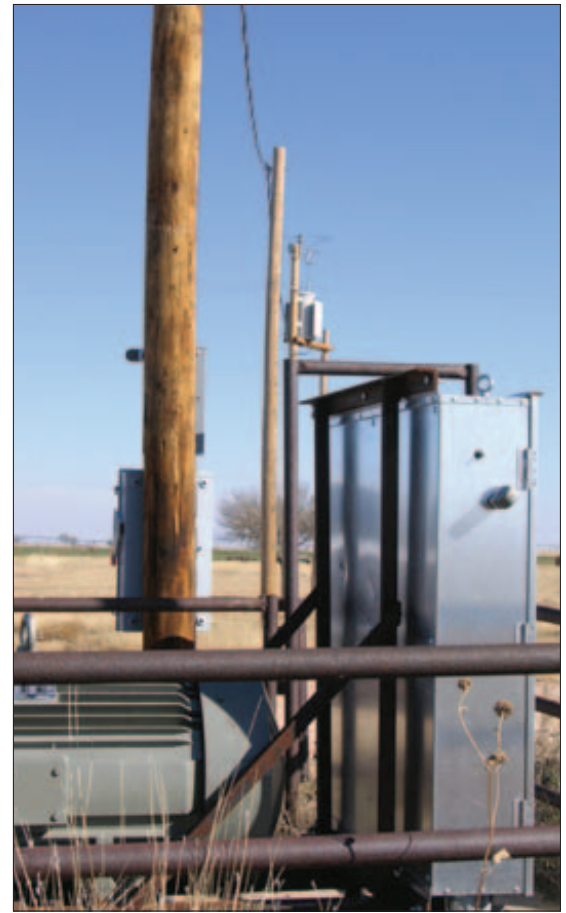
SUPPLY LINE: All the current that's needed for a 100-horsepower Written-Pole motor on David Sowers' New Mexico irrigation well comes in through a single-phase electrical line.
