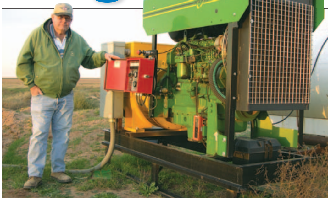
REMOTE POWER: Kenny Adams says he can use generator sets like this one to power multiple fields of irrigation in remote locations. He particularly likes generated electricity for his drip-irrigated cotton fields.
