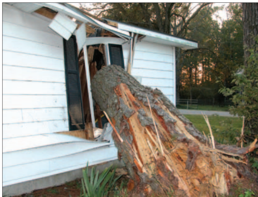
THROUGH THE ROOF: A hurricane that hit Eastern North Carolina in 2003 caused extensive damage.
