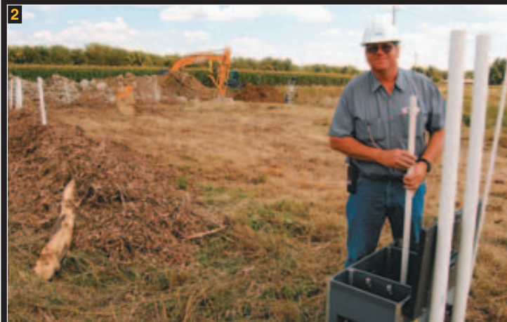
4. WATER CONTROL: Phil Algreen, Agri Drain, says, on average, one drainage control structure is sufficient for approximately 20 acres. This particular control structure is solar powered and sends updates via satellite. Landowners can control it remotely via the Internet.
