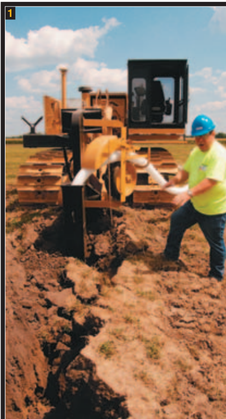
1. DIG IT DEEP: Jim Kiley of ILICA says most tile main lines are 6 to 8 inches in diameter. They feed 4-inch lines, which are controlled via underground gates. Kiley estimates tile runs $2.50 per foot, installed.
