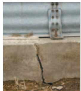
FRACTURED: Concrete grain-bin foundations crumble above subsiding soil.
