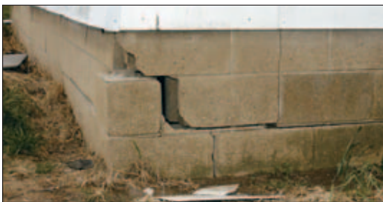
CRUMBLING: Foundation cracks are not unusual results of longwall mining subsidence.
