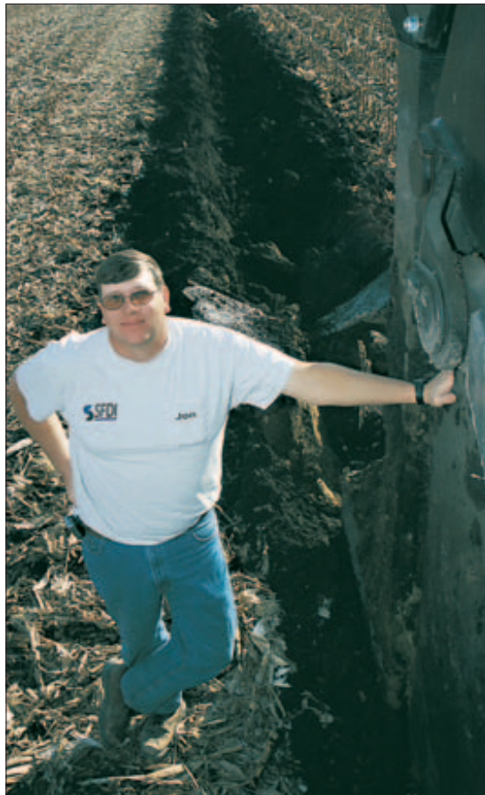
HEFTY START-UP: Laying tile requires a healthy machinery investment, says Jon Seevers, who runs a $300,000 self-propelled, laser-guided tile plow.
