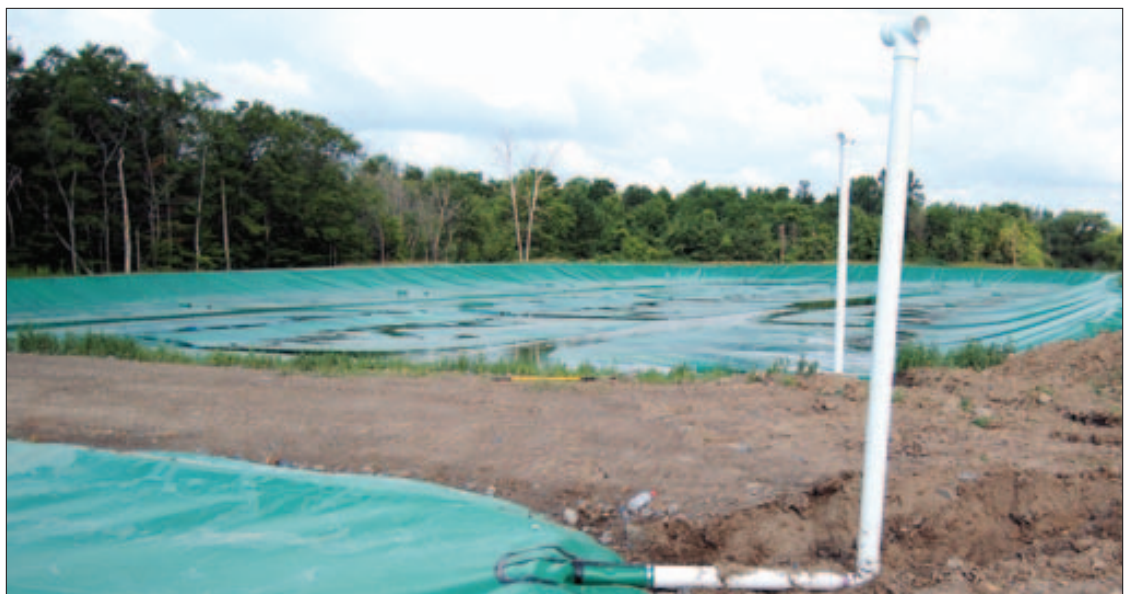
CARBON CAP: Fessenden Dairy is installing this polymer lagoon cover as a manure odor reducer at no cost to the Fessendens.
